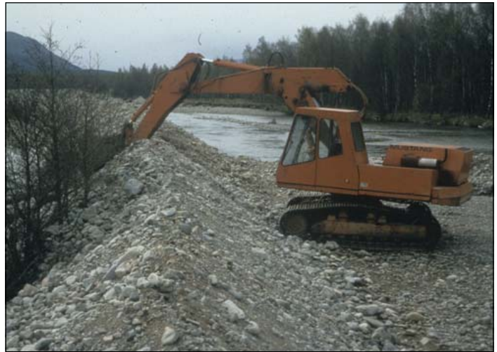
Digging a diversion channel in the Feshie fan. The river in flood soon removed the masses of boulders and gravel built up.
