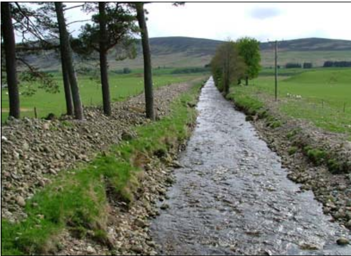
River “management” in Glen Clova. A digger has been used to take gravel from the river bed, leaving the river ecology badly damaged, to produce a rather ineffective flood barrier.
